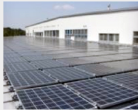
Solar power - 60 kw (Fukuroi Factory, Japan)
