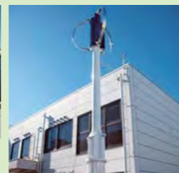
Vertical wind power generation system, which is quieter than the propeller type (Nakaze Factory)
